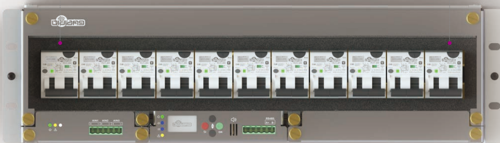
Macro site Solution 8: Multi communication network (5G) / multi operator (with metering sub-load)
